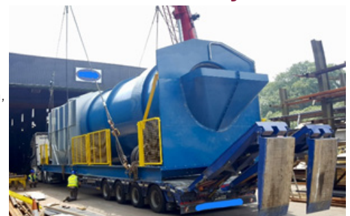
Installation of the pulper, a key part of the process to turn mixed waste paper back into a salable pulp.
