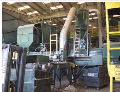
Victor Valley MRF, located in Victorville, CA
